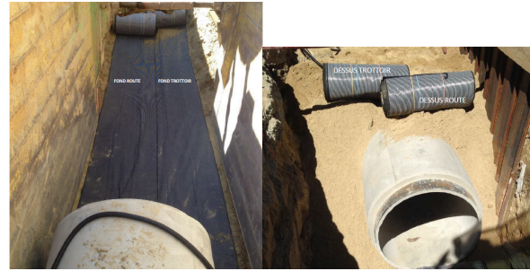
Figure 3: Sensor-enabled geotextile placed below and above the pipeline.
